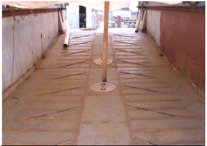
New Cargo Deck installed with hatches so that we can access the under deck voids for inspection and cleaning, note new diagonal traction strips which will not pool water
