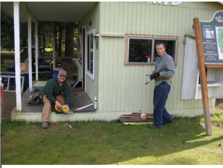
Rusty and Less installing new windows and doors on the Starter Shack, looks like more fun than work!
