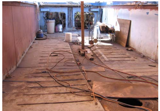
View of Elsie M II from Bow, looking aft showing new deck being welded in place.
