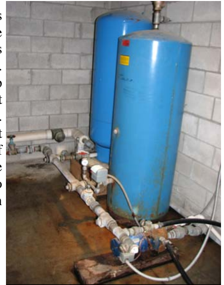
G Tank before repair
